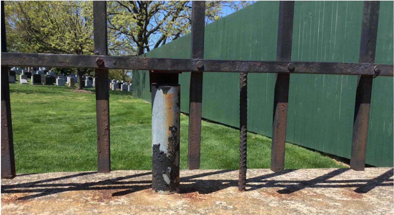
Figure 35- Pipe Support at Fence
