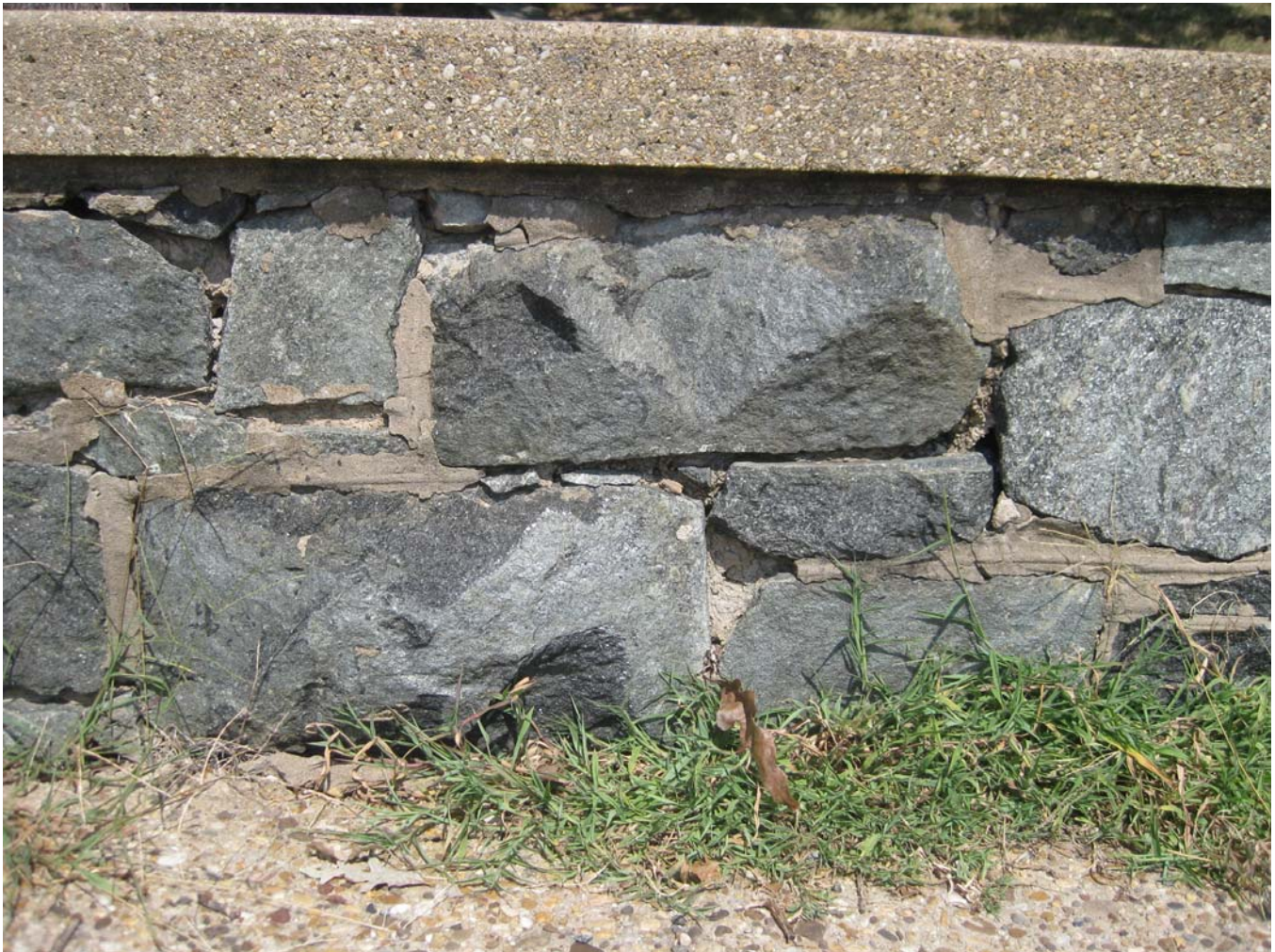
Figure 33- Deteriorated Mortar (typical view from outside cemetery)
